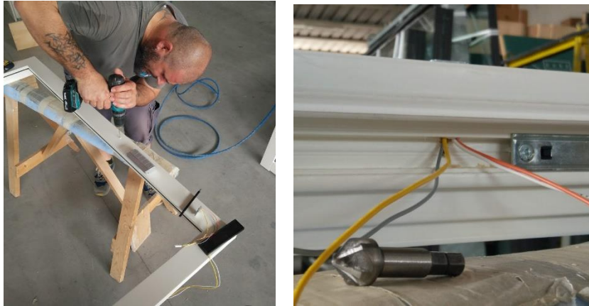
Figure 8. Shading system electrical installation (Source: Eurofinestra)
